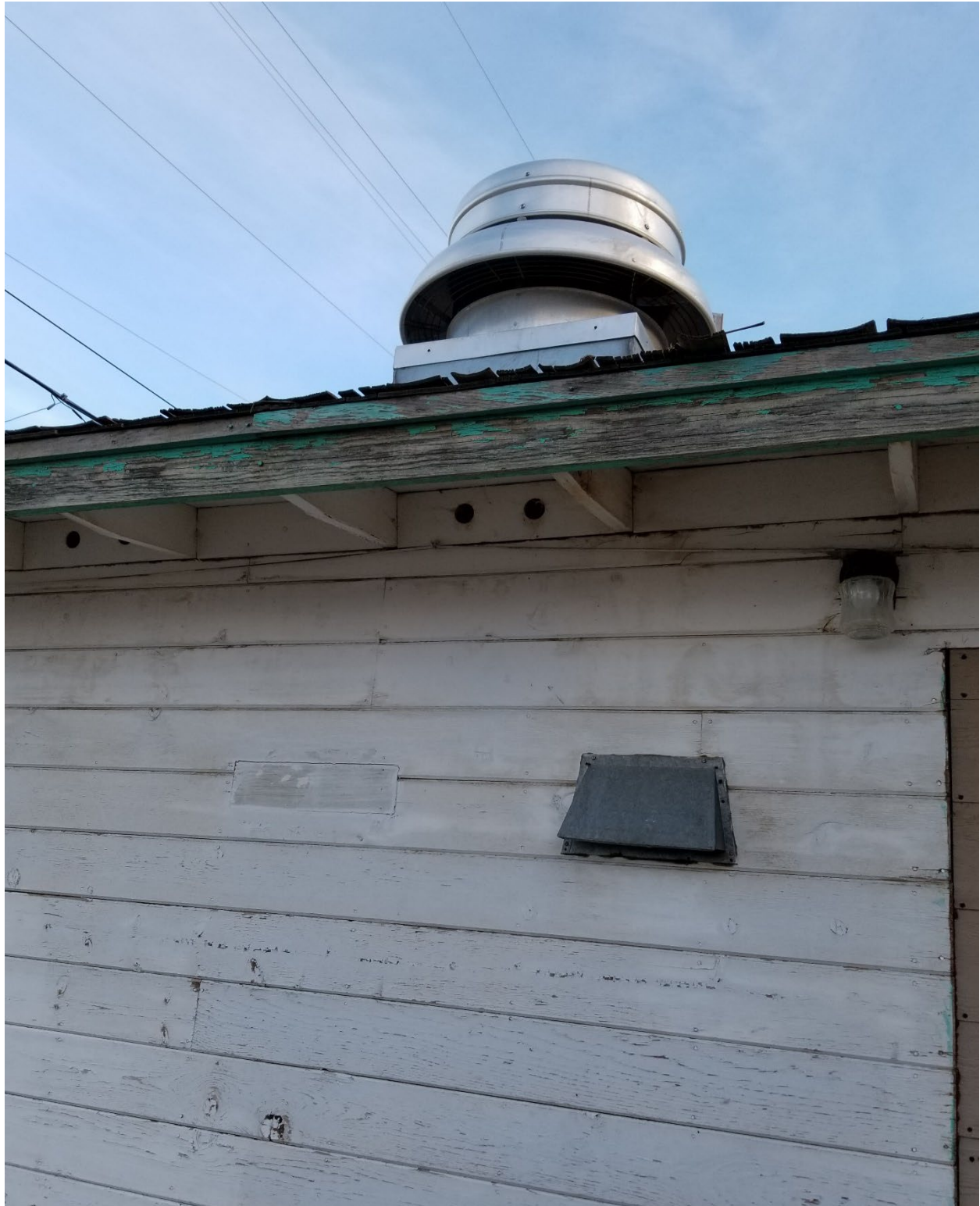
Figure 6. Roof vent hood for the V.O.C.A. building.
