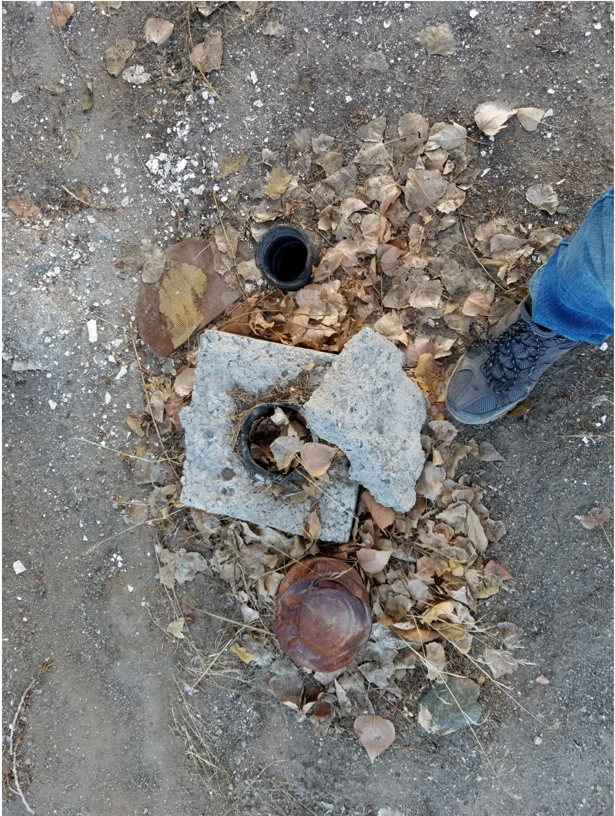
Figure 5. Sewer or septic cleanout located near the exterior of the V.O.C.A. building.
