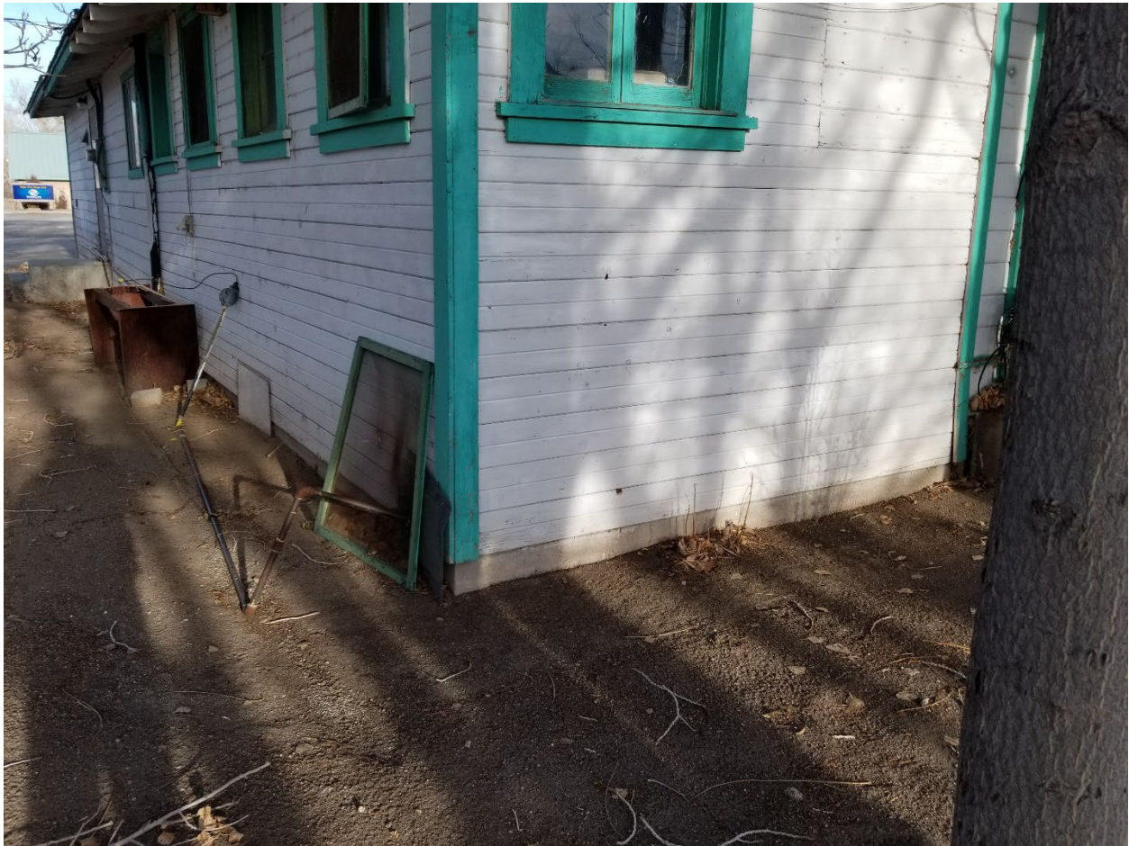
Figure 4. Northwest exterior side of the V.O.C.A. building showing the propane regulator.
